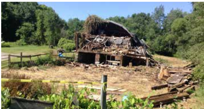
Part of the same structure collapsed during the winter and is being torn down. Now owned by Cathy White. August 2015
