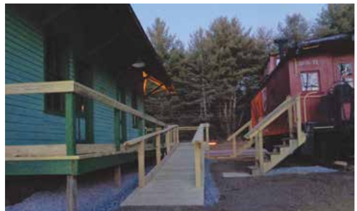
Work was done on the Caboose and Train Station in October and November 2021. The ramp was put in by the Boy Scouts.
